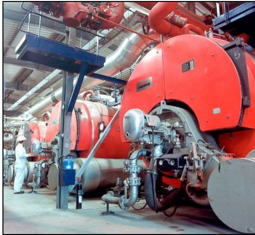
Example of a gas-fired back up boiler station
